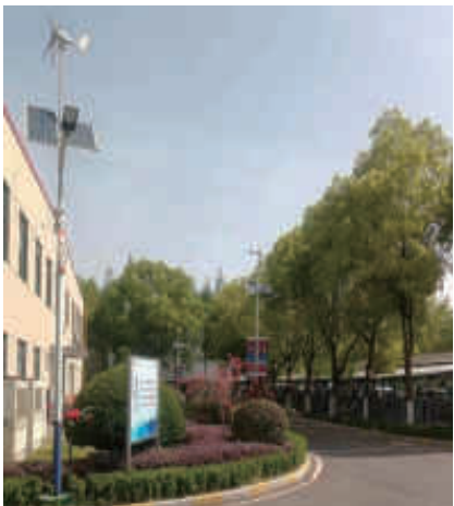
Wind-Solar Complementary Solar Street Lights
