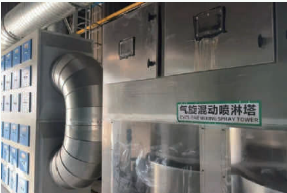
Exhaust Gas Treatment Facilities
