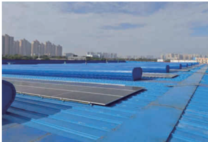
Rooftop Photovoltaic System
