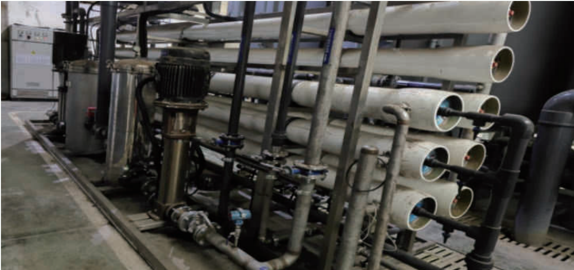
Recycled Water Reuse Membrane Modules
